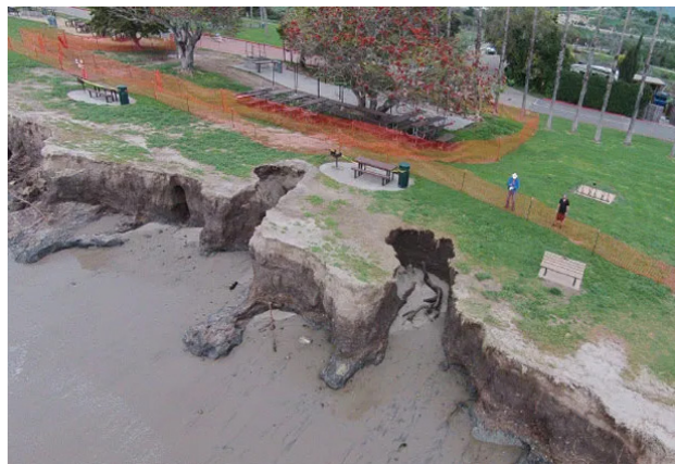
Figure 20: Major erosion from winter storms at Goleta Beach County Park. Photo Source: Arthur Sylvester, Noozhawk , 2016.
